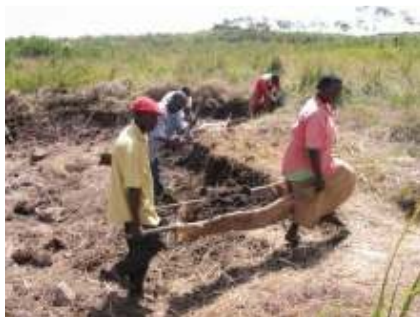
5: Dig the soil from the dig areas and move it to the fill areas (Mbugua H. M.)
