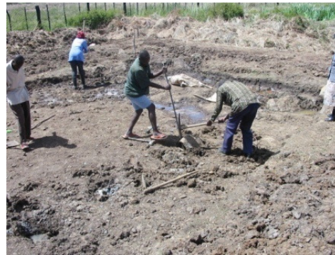
6: Make sure that you remove all boulders and tree stumps from the pond area (Mbugua H. M.)
