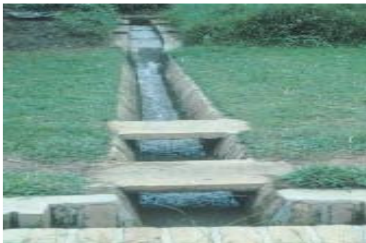
15: An open water supply canal lined with concrete slabs (Ngugi C. N.)
