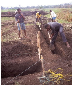
8: Where soils are too pervious, dig a trench all round within the dyke position before constructing the dykes (Ngugi C. N.)
