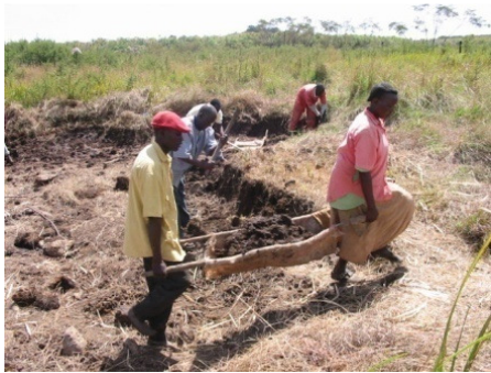
5: Dig the soil from the dig areas and move it to the fill areas (Mbugua H. M.)
